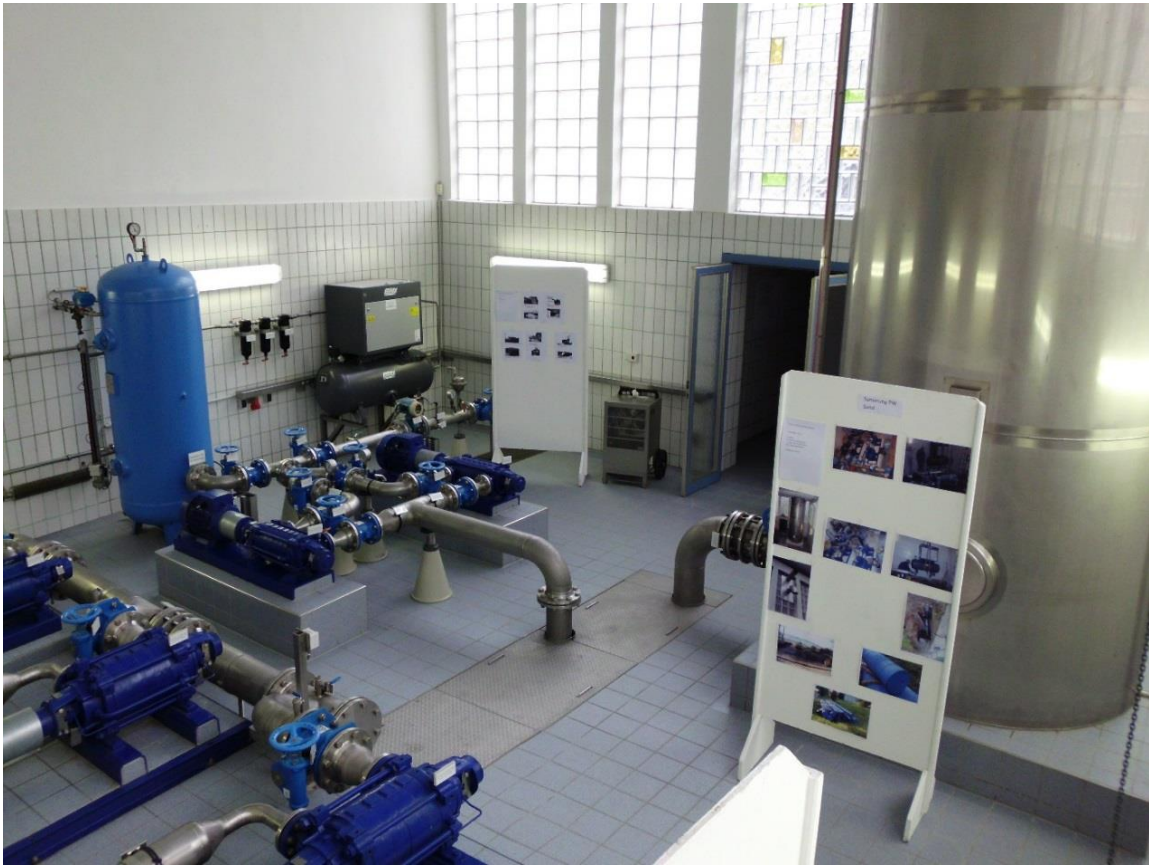
Blick in das Pumpwerk
